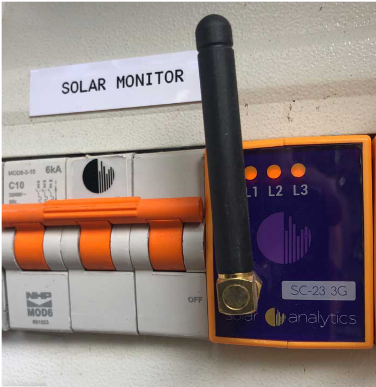
A consumption monitor in my switchboard.
